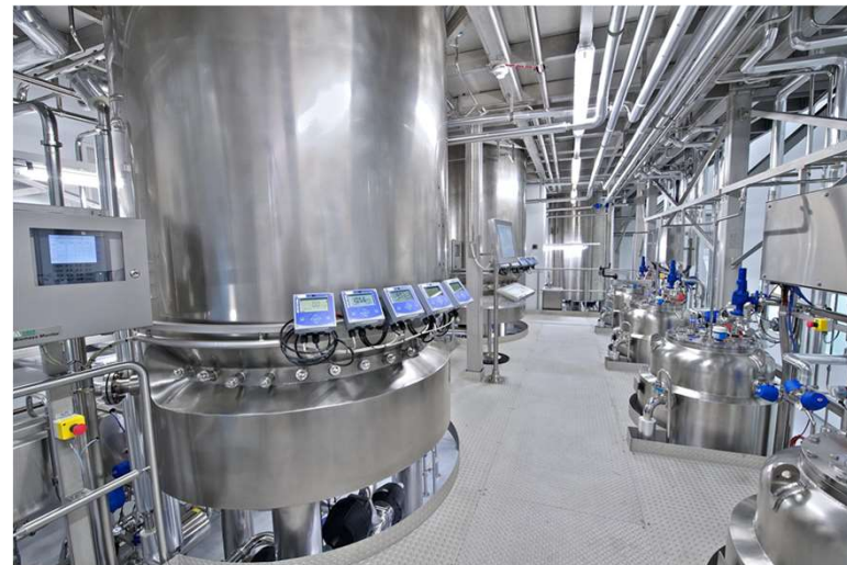
Food factories - Cooling/Heating
