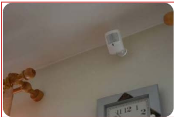
Detectors in flats
