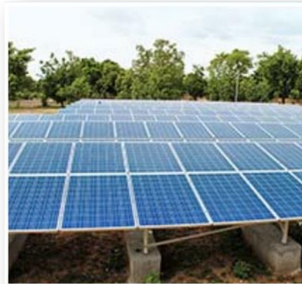
Asantys Systems has installed 550 kWp in Solar-Diesel Hybrid Village Power Systems in Mali
