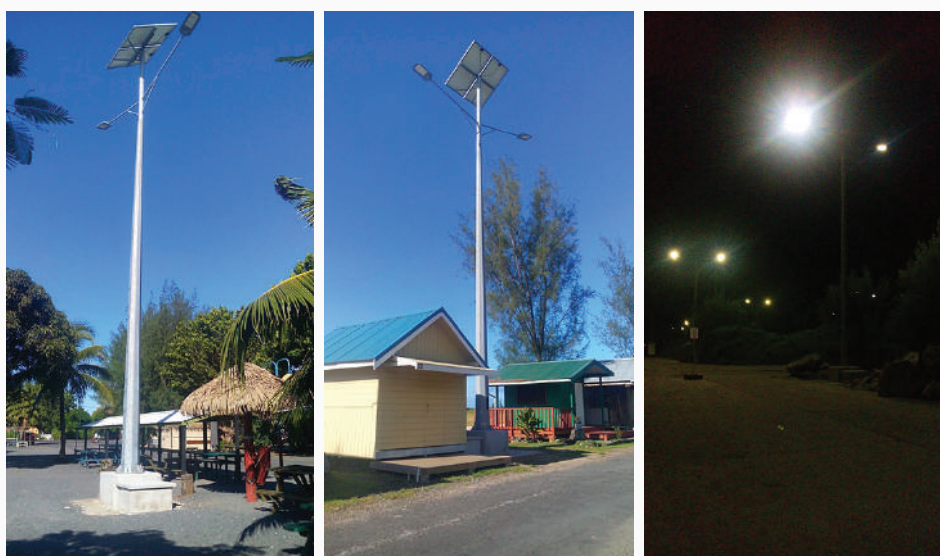
Figure 5.54: Solar/LED Lighting System at Punanga Nui Market
