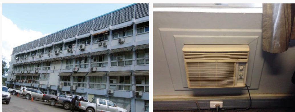
Figure 5.57: Existing AC Units at MFEM
