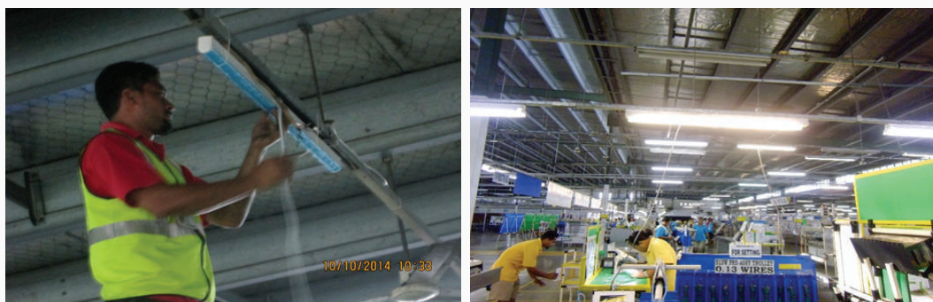
Figure 5.92: Lighting Installations at Yazaki
