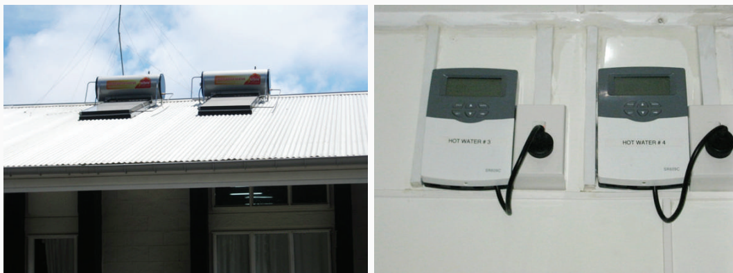
Figure 5.97: Solar Water Heaters and Monitors Installed at Medical Ward
