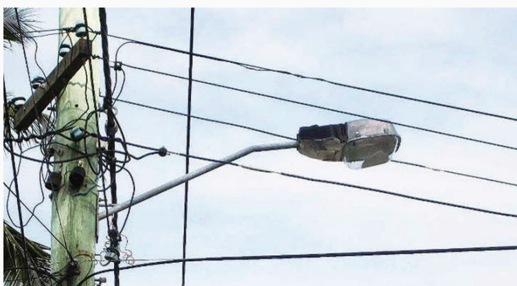
Figure 5.73: Typical HPS Street Lighting in Ha'apai, Tonga
