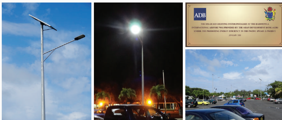
Figure 5.52: Solar/LED Installations at the Airport Car Park
