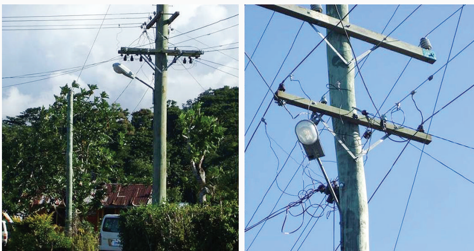
Figure 5.68: Current MV Luminaires in Apia, Samoa
