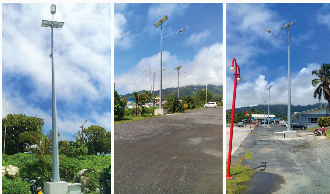
Figure 5.63: Solar/LED Lighting System at the Marina & Wharf – Cook Islands
