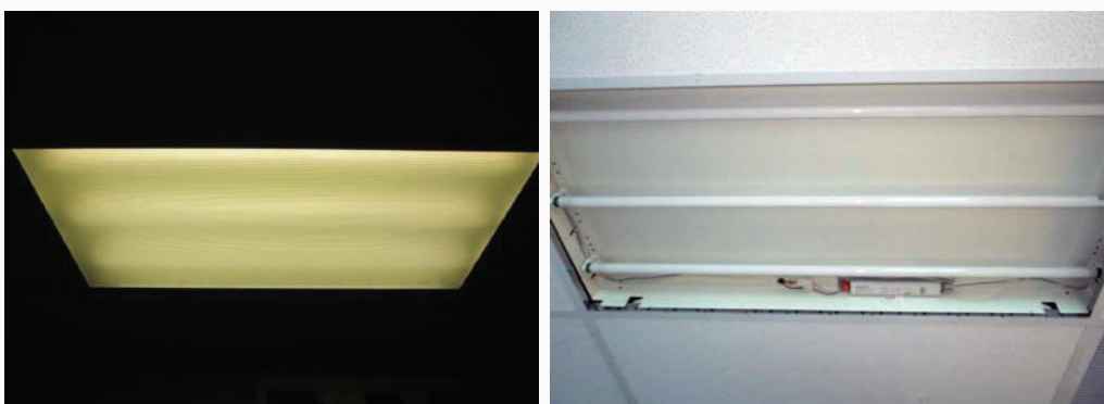
Figure 5.87: Current Luminaires at DBS building
