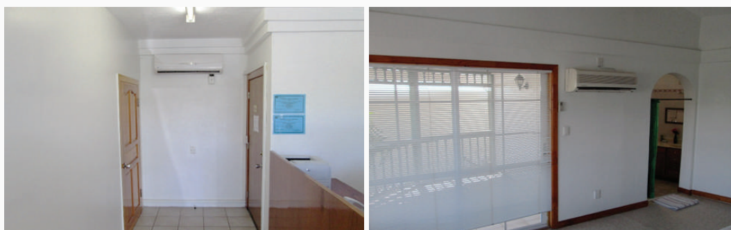
Figure 5.93: AC Installation at Pacific Pearl Hotel
