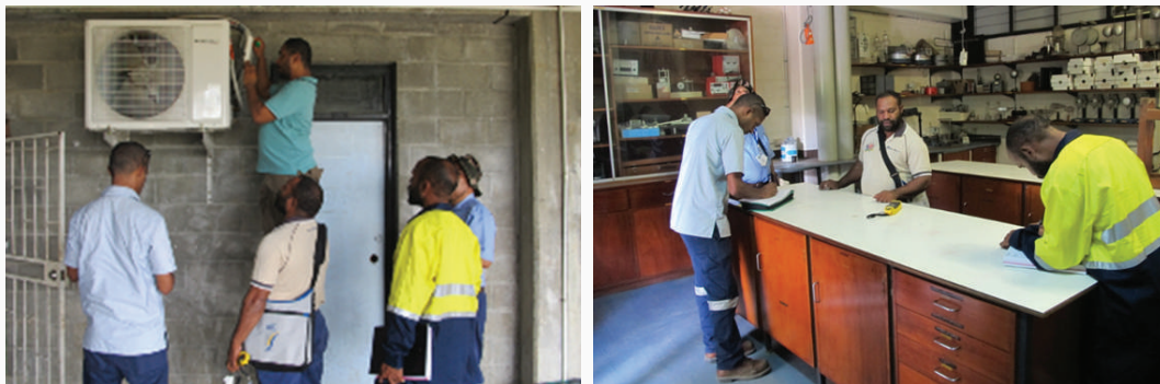
Figure 5.38: M&V Activities for A/C and Lighting Systems Conducted in UPNG
