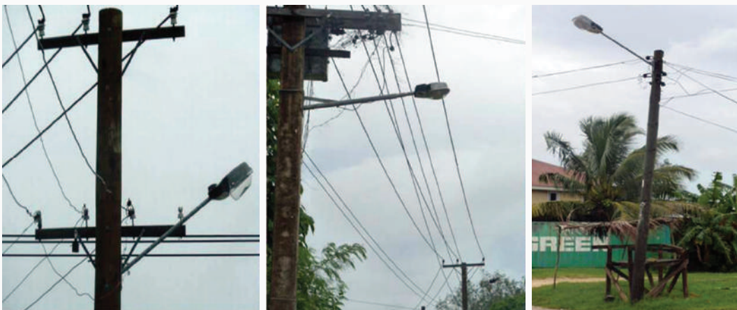
Figure 5.74: Typical HPS Street Lighting in Tongatapu, Tonga
