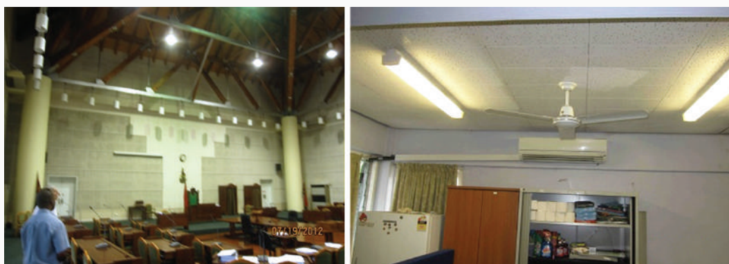
Figure 5.67: Existing Lighting in the Parliament and National Statistics Office
