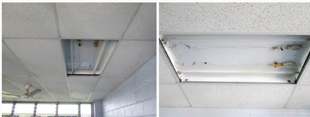
Figure 5.86: Current Luminaires at NUS
