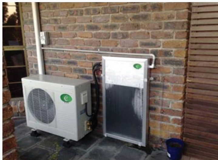
Figure 5.90: Example of Solar Hybrid Air Conditioner
